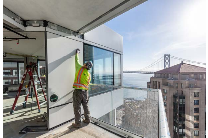
Permasteelisa handled the fabrication and installation of the facade, wrapping up a floor approximately every four days. In total, there are over 4,700 curtainwall panels. (Jason O’Rear)
